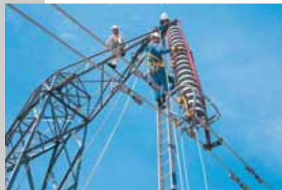
Utilities and process control centers
